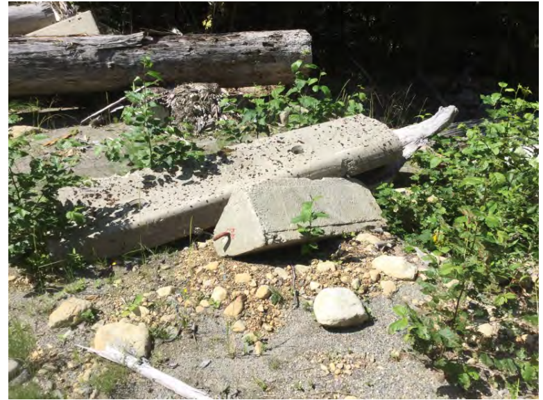
Transition and bullnose not attached upstream left approach
