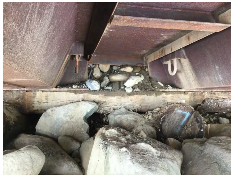
No ballast wall at left bank
