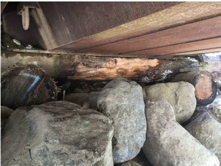
Face logs were never completely peeled and minor sap rot noted
