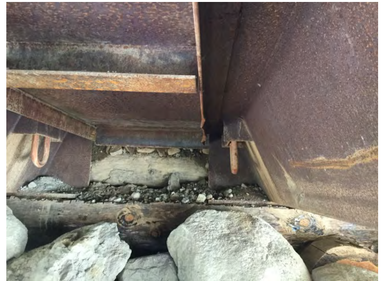
Bridge guide angle deformed at upstream right bank
