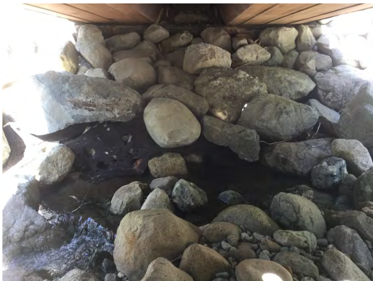
Right Bank Abutment when facing downstream, scour noted
