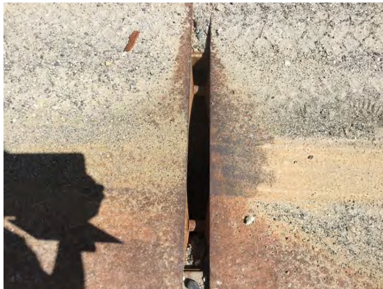
Spacer plate is constructed in 2 pieces and steel at joint has started to deform, no timber blocking
