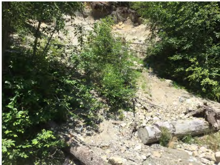
Ravelling cutbank at right approach
